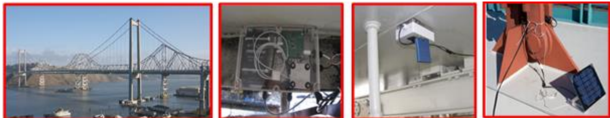
Figure 3-5: structural health monitoring components
